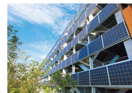
Solar panels LaLaport IZUMI
